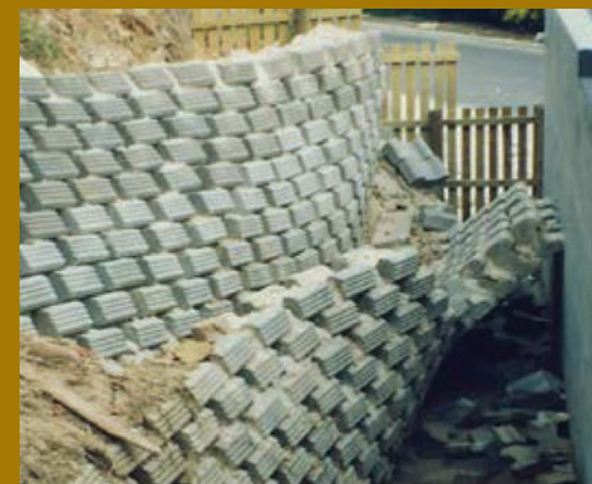
Incorrect stability calculations and limited bearing capacity, resulting in overturning
