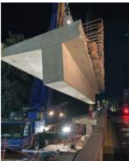
A precast T-beam is lowered into position by two mobile cranes. (Image supplied by Edward Smuts).
