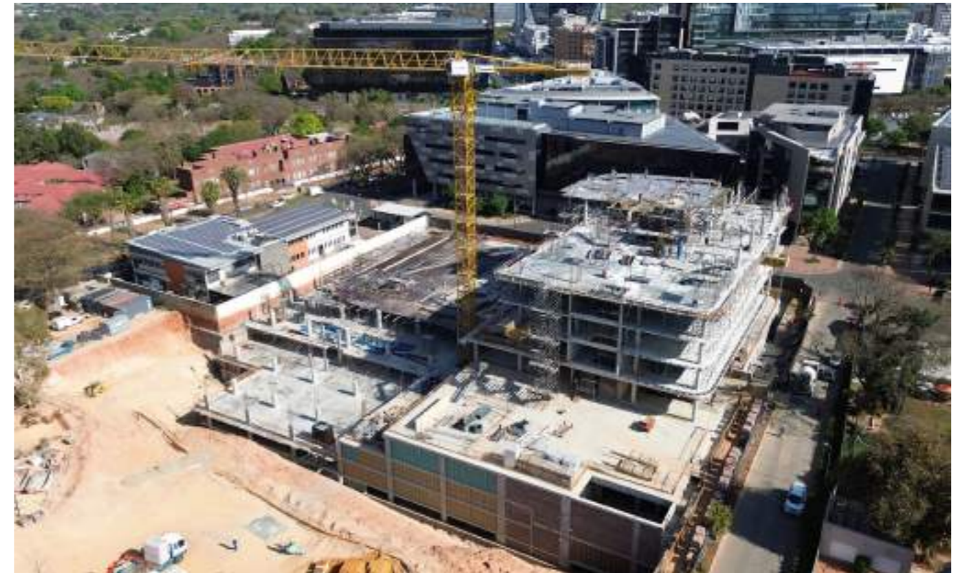
The common basement of 10 Parks Boulevard and 55 Eastwood Road is a substantial structure, utilising 15,350 cubic metres of concrete and 1,620 tonnes of rebar.
