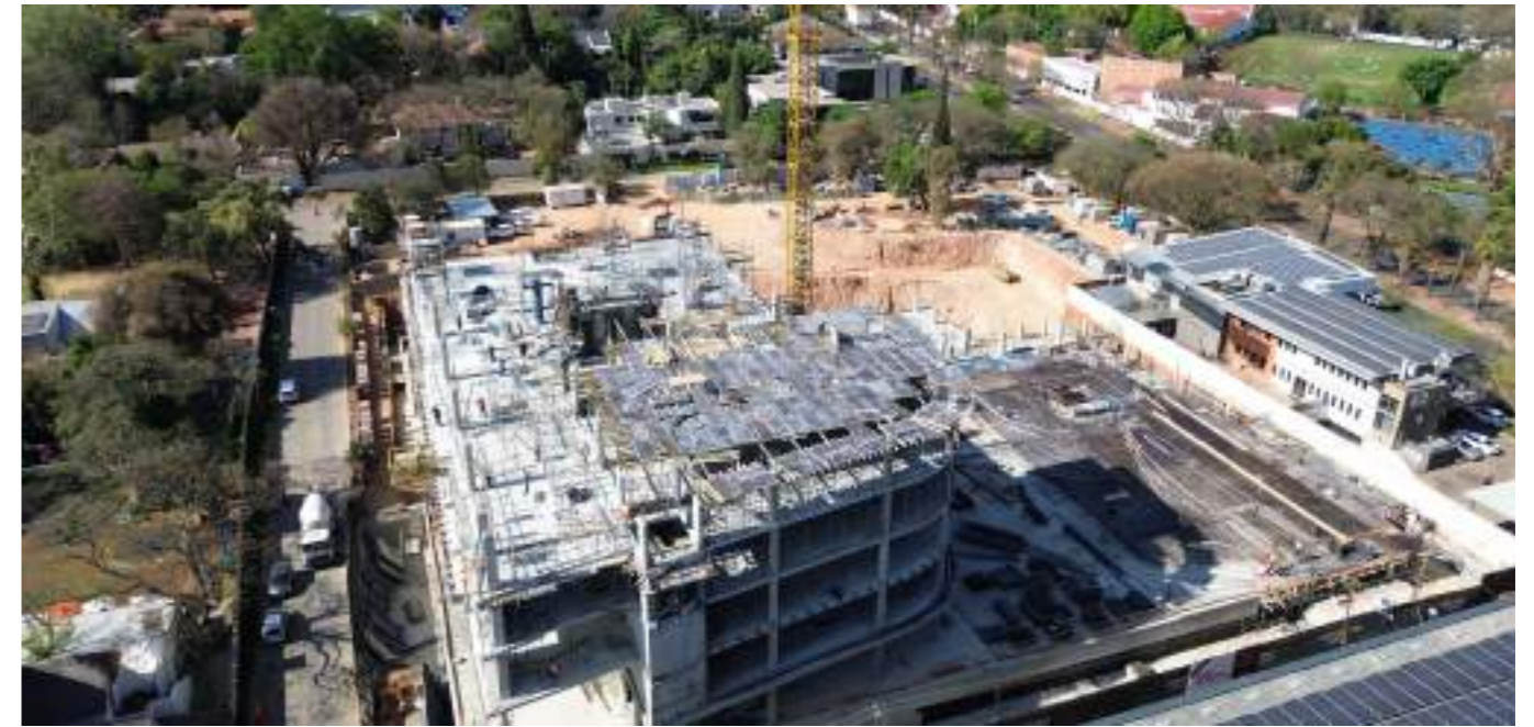
10 Parks offers five floors of office space and a retail floor totalling 7562m 2 GLA, while 55 Eastwood provides three floors of office space and a retail floor covering 4734m 2 GLA.
